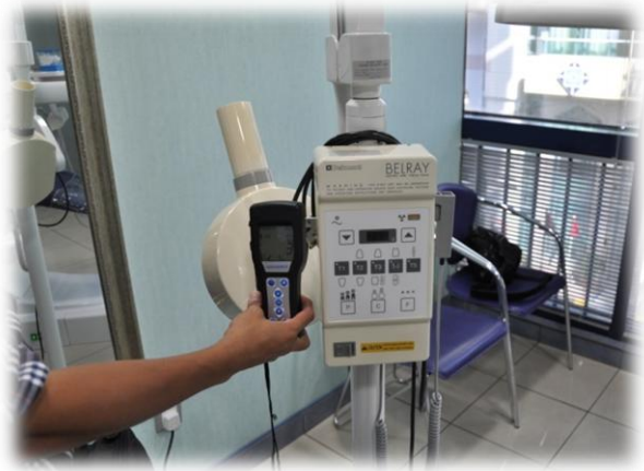
Control panel @ 3-safe
