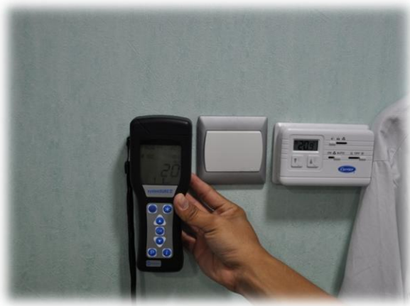
Switches of the Operation room @ 20-caution
