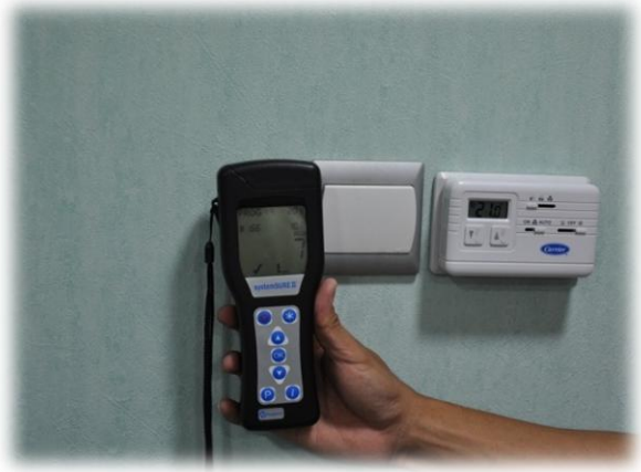
Switches of the Operation room @ 7-safe
